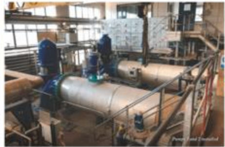
Pumps and Electrical
